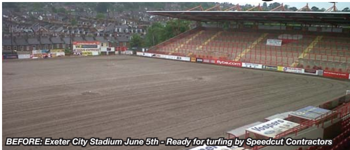
BEFORE: Exeter City Stadium June 5th - Ready for turfing by Speedcut Contractors
