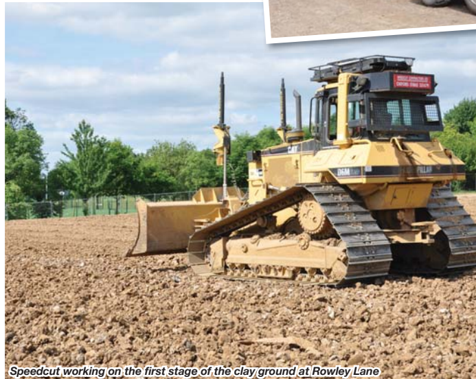
Speedcut working on the first stage of the clay ground at Rowley Lane
