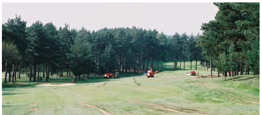
Extensive drainage work carried on the Longcross course at Foxhills in late spring before the heavy rain
